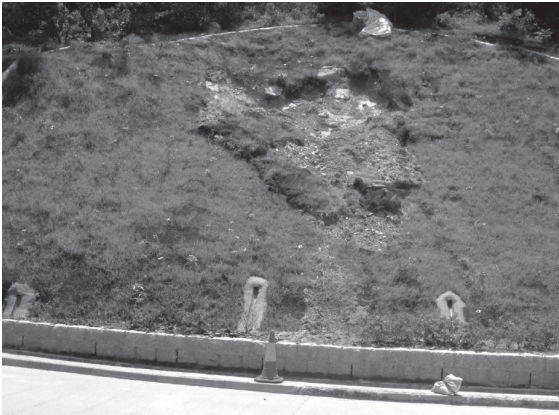
Figure 29. Shallow failure at a completed soil-nailed slope
