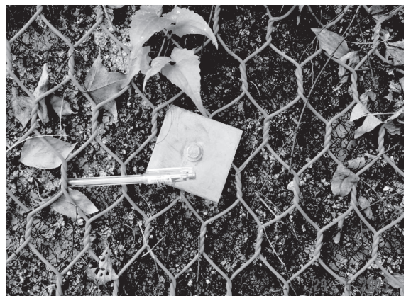
Figure 7. Details of the use of steel wire meshes in conjunction with non-degradable erosion control mats
